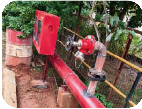
FIRE HYDRANT SERVICE
