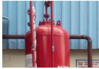
FOAM BASED SPRINKLING SYSTEM
