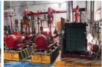
PUMP HOUSE SYSTEM
