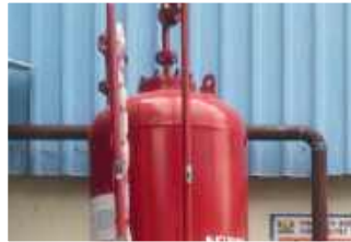
FOAM BASED SPRINKLING SYSTEM
