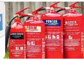
FIRE EXTINGUISHERS AND SAND BUCKET
