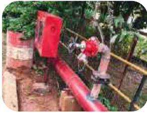
FIRE HYDRANT SERVICE
